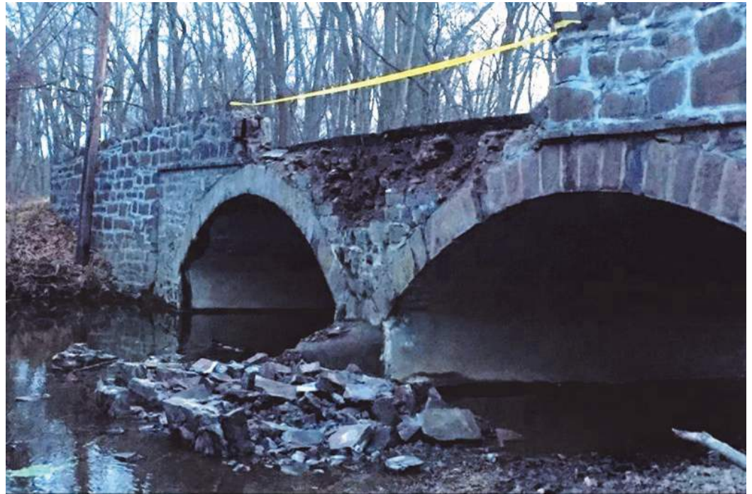
Bridge on Keith Valley Road damaged by one-car, non-fatal accident on December 21, 2015. (photo courtesy of Horsham Twp.)
